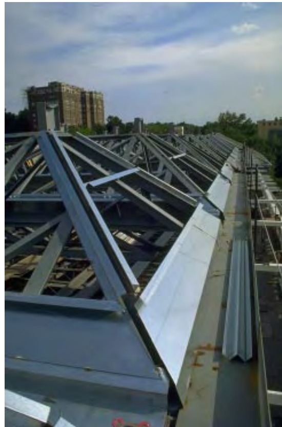
Nucor-Yamato 100% recycled steel; Prefabricated modular trusses & columns
